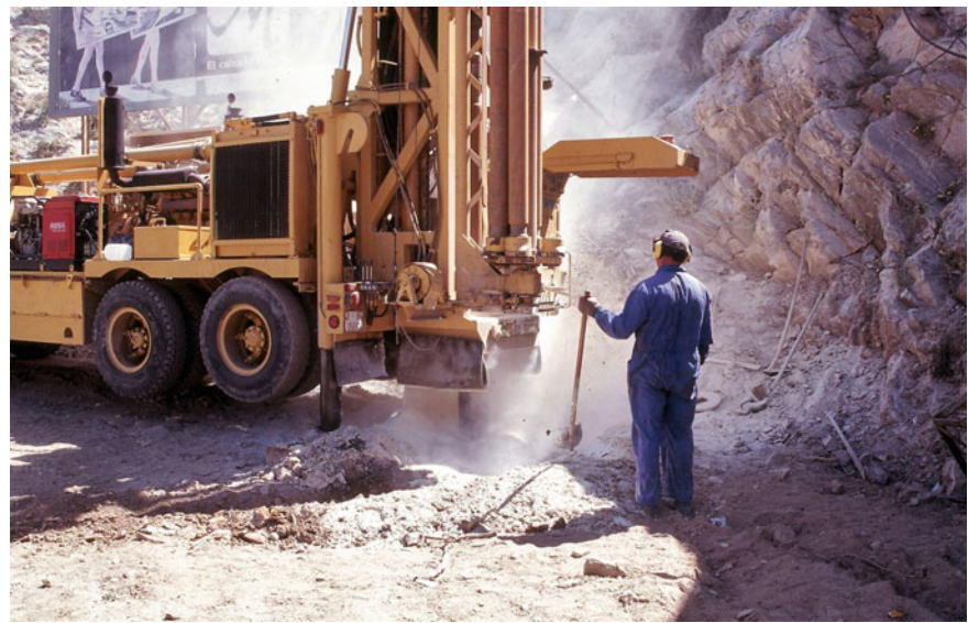
Photo 8.13 Rotary-percussion machine sinking a borehole in the marble of Castell de Ferro (Granada) (Photo A. Pulido)
