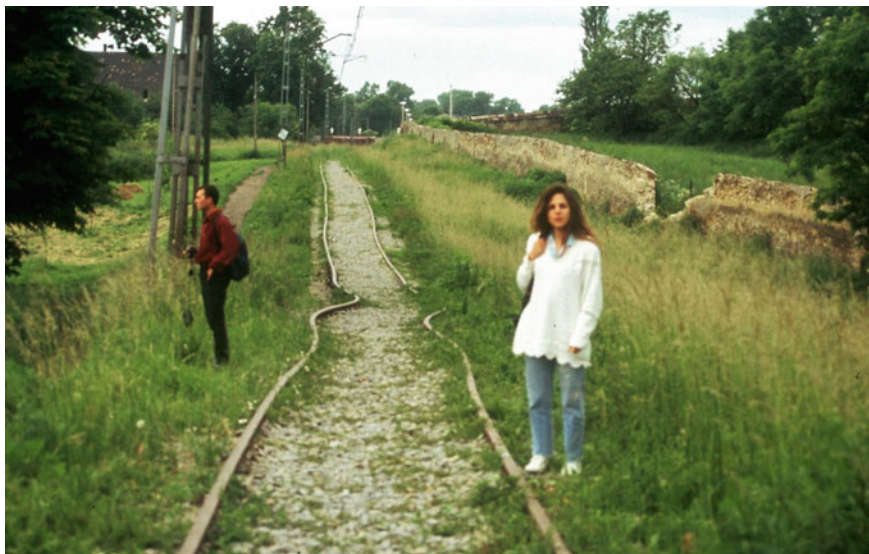
Photo 8.21 Deformed rails and broken walls as a result of settlement in the vicinity of the Wilyzca mines (Poland) (Photo A. Pulido)
